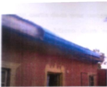
Plate 3: Informal RWH Design Source: Field Survey 2018
